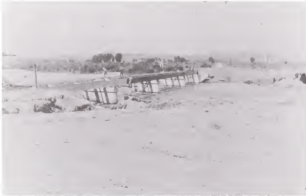
The final stage of construction included the addition of the floor beams and braces before the deck was emplaced. This bridge is located approximately five miles north of Belfry on Montana Highway 72 (Robbins Photograph).
